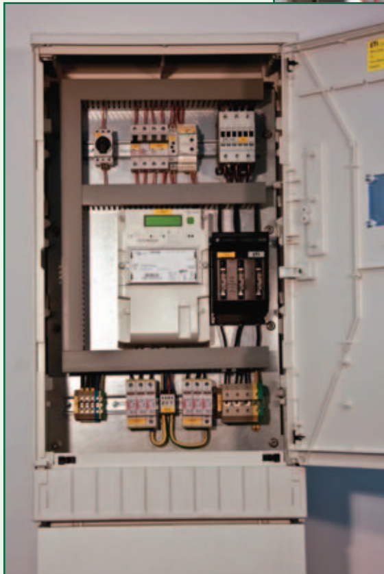
Meter distribution cabinet
